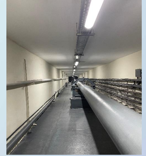
Experimental hall at IREN facility
