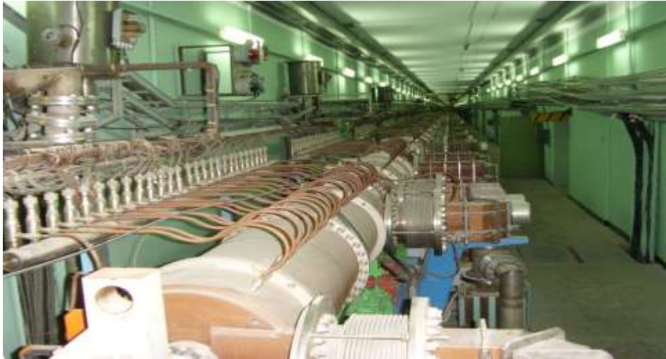
Fig.8. Basic part of the accelerator ( f=991 MHz). The total length of the accelerating structure is 360 m.
